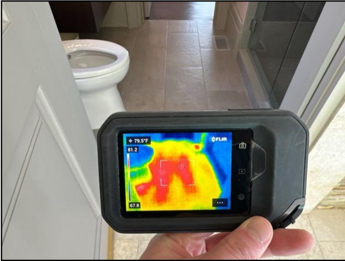
Hot water radiant piping
