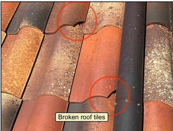
Missing, loose or broken pieces
