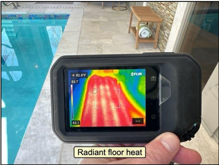
Hot water radiant piping
