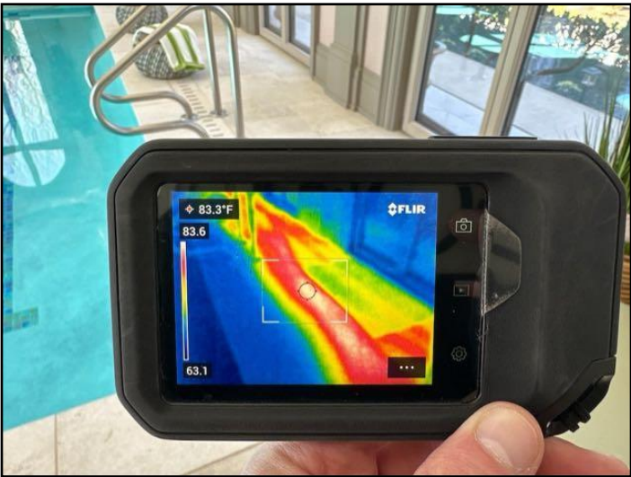
Hot water radiant piping
