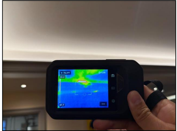
General view of cooling system
