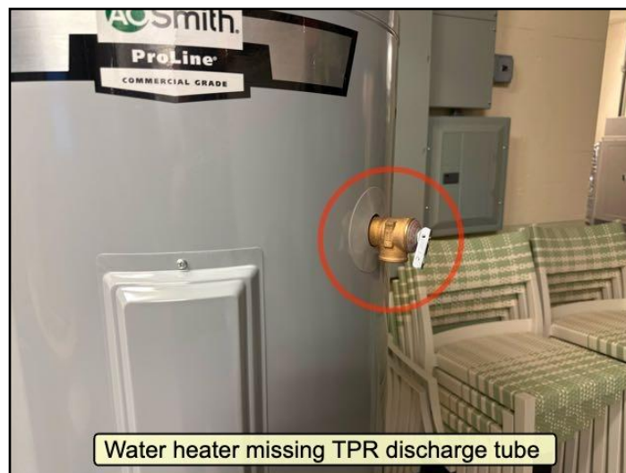
Discharge tube missing
