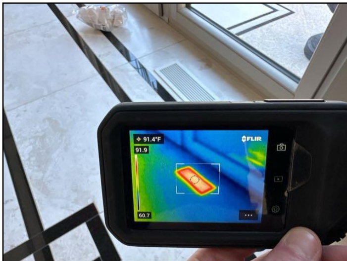
General view of heating system
