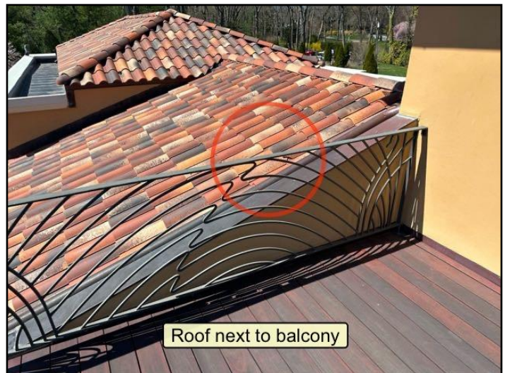
Missing, loose or broken pieces
