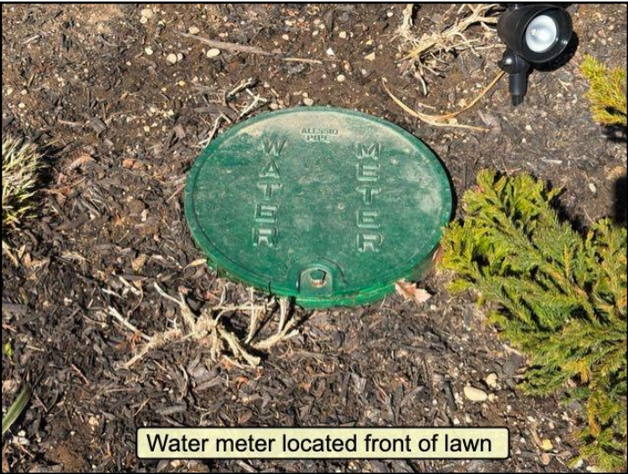
Water Meter outside front lawn
