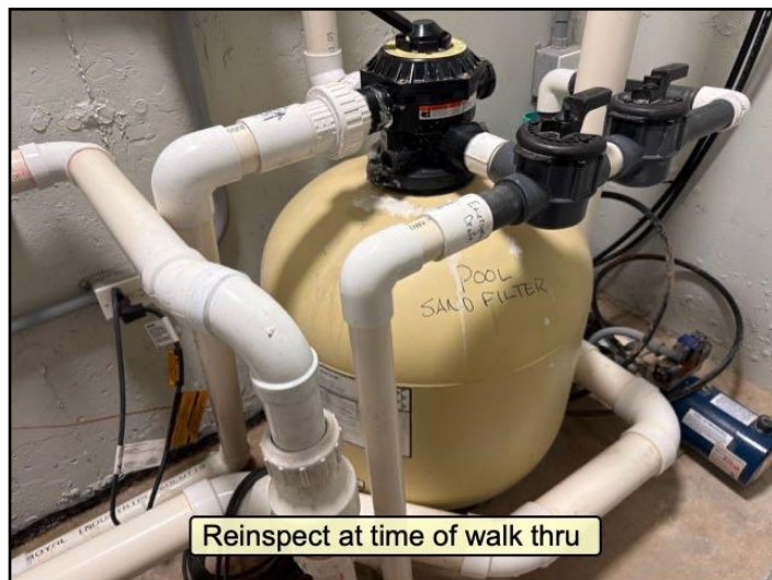
General view of pool and equipment
