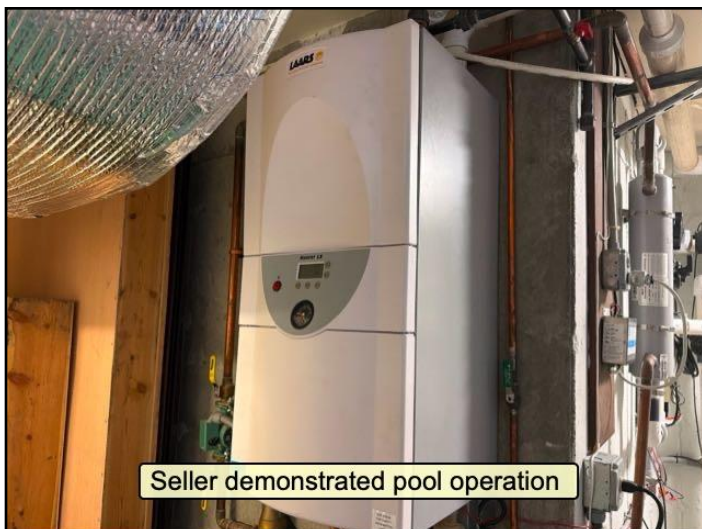
General view of pool and equipment
