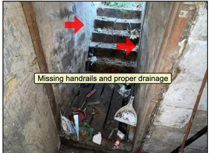
Masonry or concrete cracking
