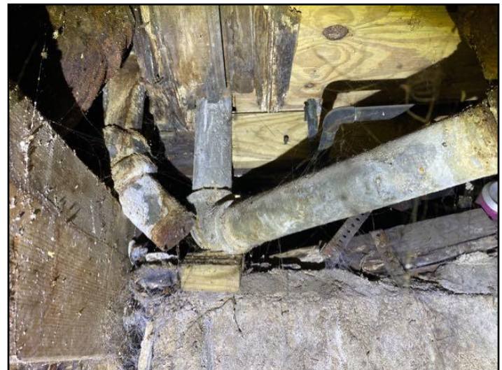
Old galvanized pipes rust from inside out...
