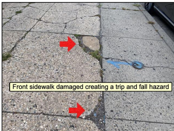
Cracked or damaged surfaces
