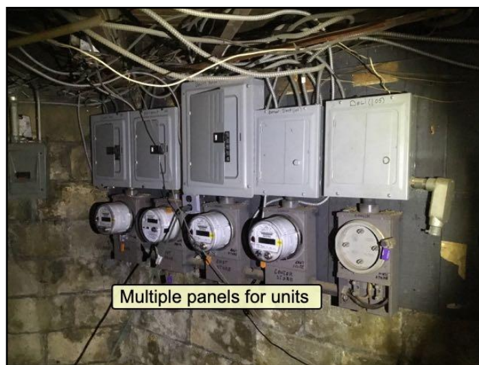
General view of electrical system
