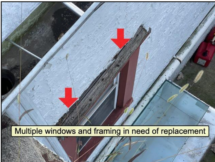
Flashing loose, missing or deteriorated
