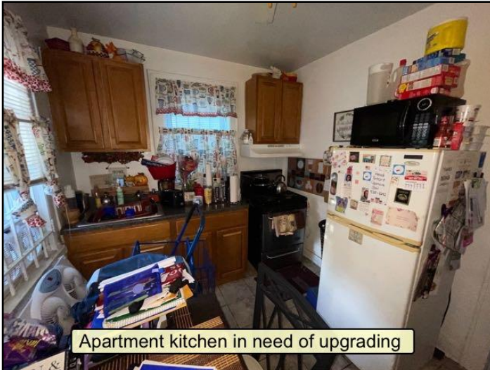
Kitchen in need of upgrading
