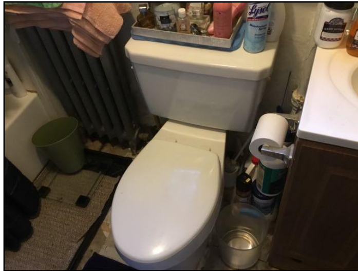
Bathroom in need of upgrading. Recommend...
