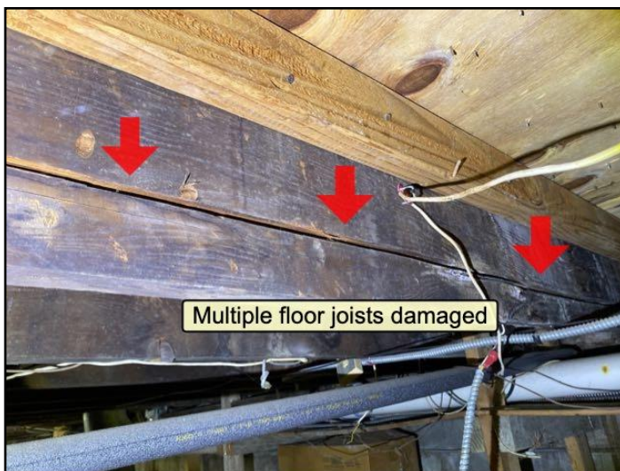
Split or damaged
