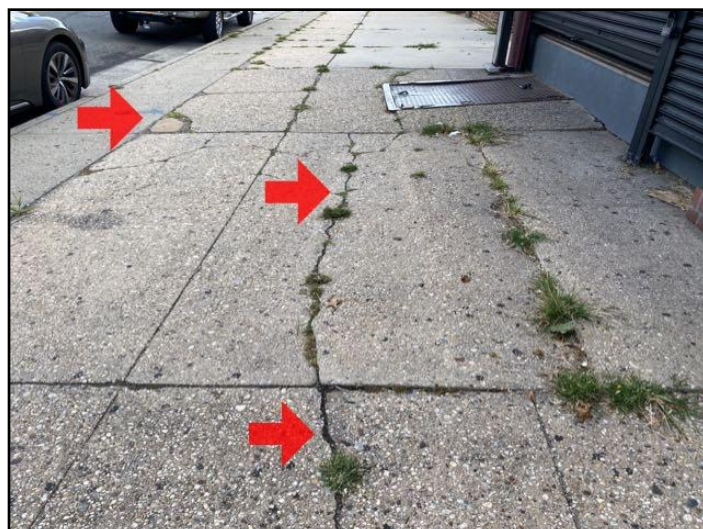
Cracked or damaged surfaces
