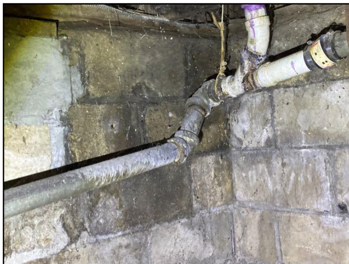
Old galvanized pipes rust from inside out....
