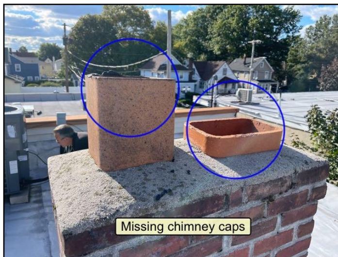
Missing chimney cap
