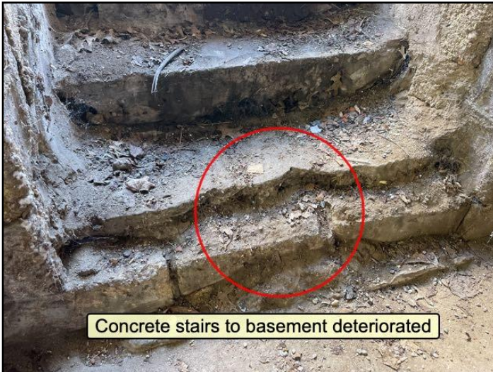
Masonry or concrete cracking
