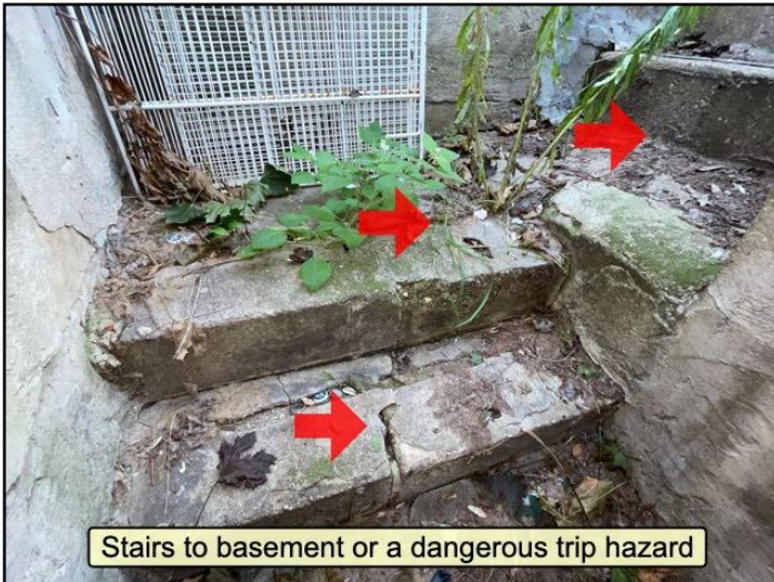
Masonry or concrete cracking
