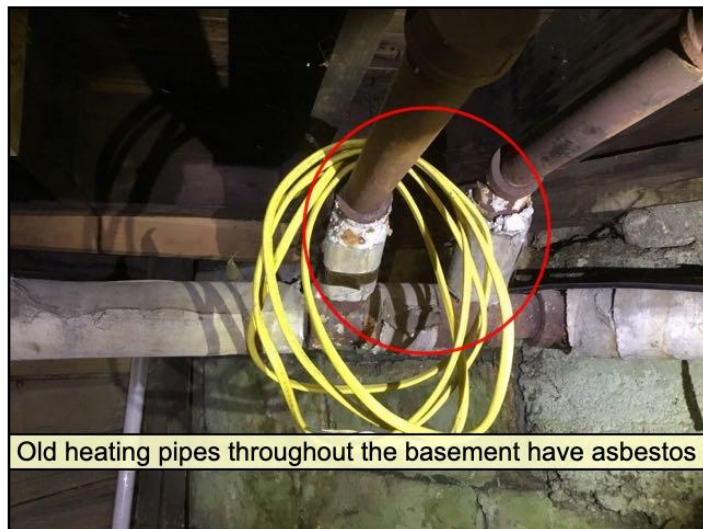
Old steam pipes may have been insulated wit...
