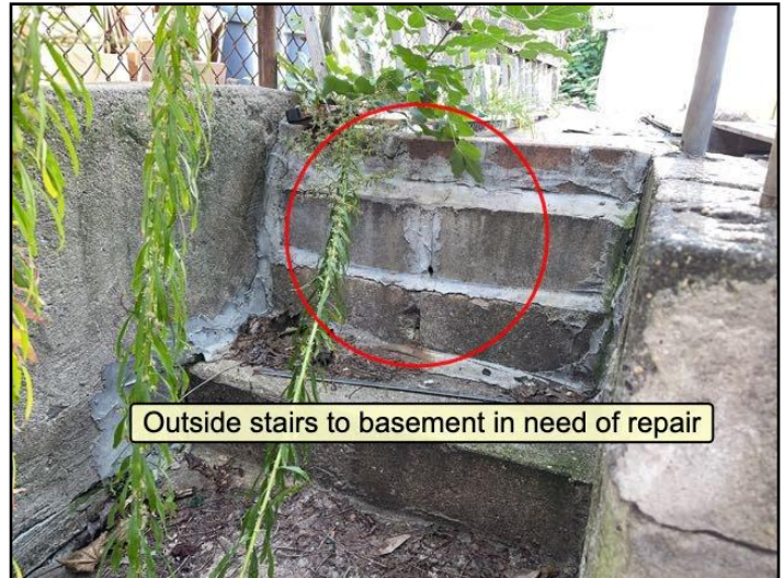
Masonry or concrete cracking
