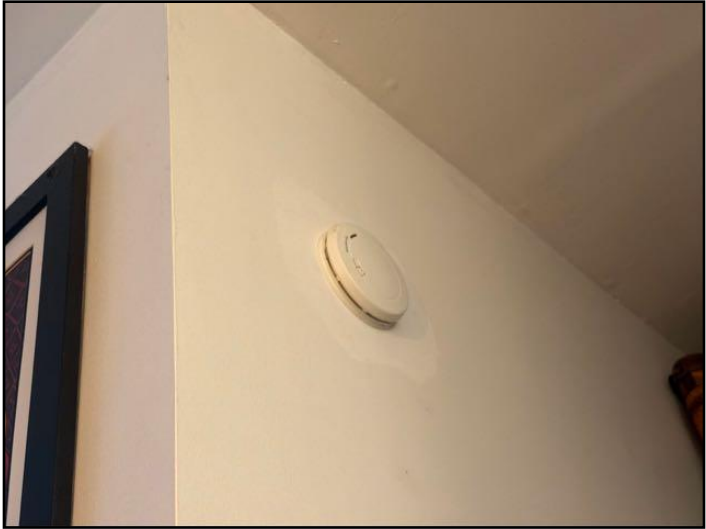
Recommend testing all Smoke and CO detectors
