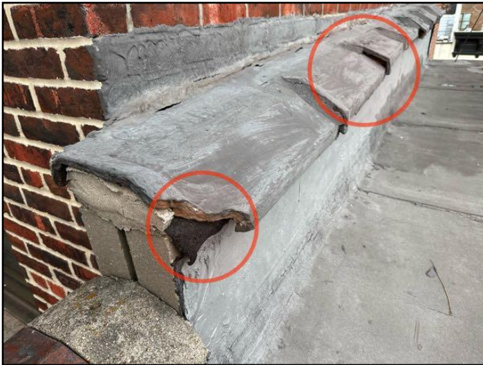
Parapet wall coping damaged
