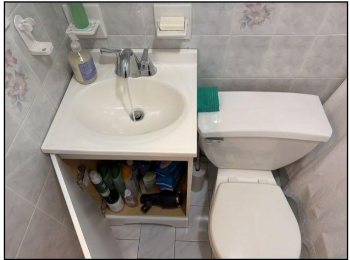
Temporary plumbing materials
