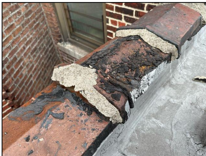
Parapet wall coping damaged
