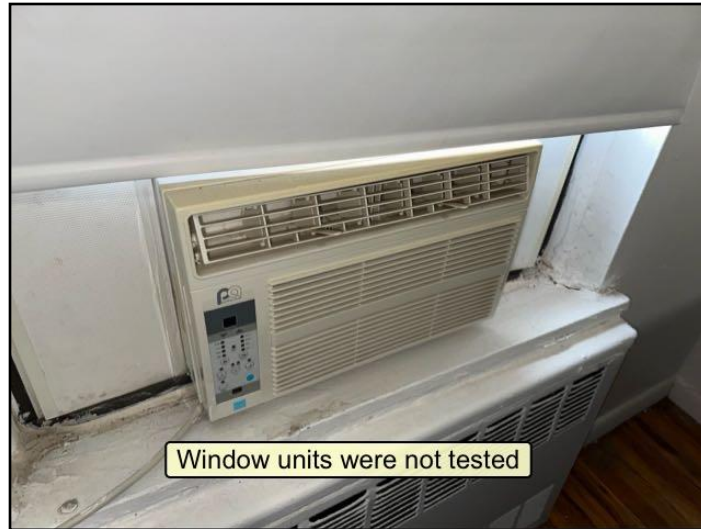
Window and wall mounted Air Conditioning...
