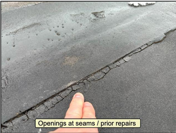
Openings at seams or flashings
