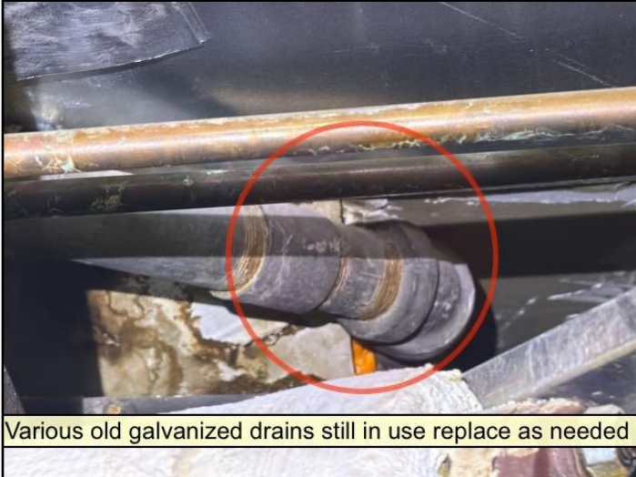
Old galvanized drains
