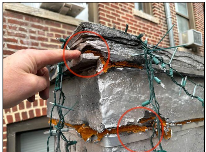
Parapet wall coping damaged
