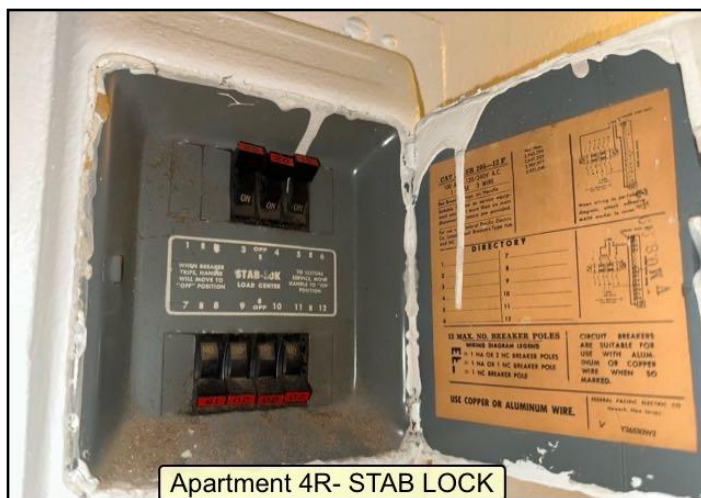
Budget for replacement of outdated / safety concern panels
