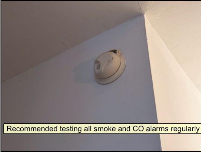
Recommend testing all Smoke and CO detectors
