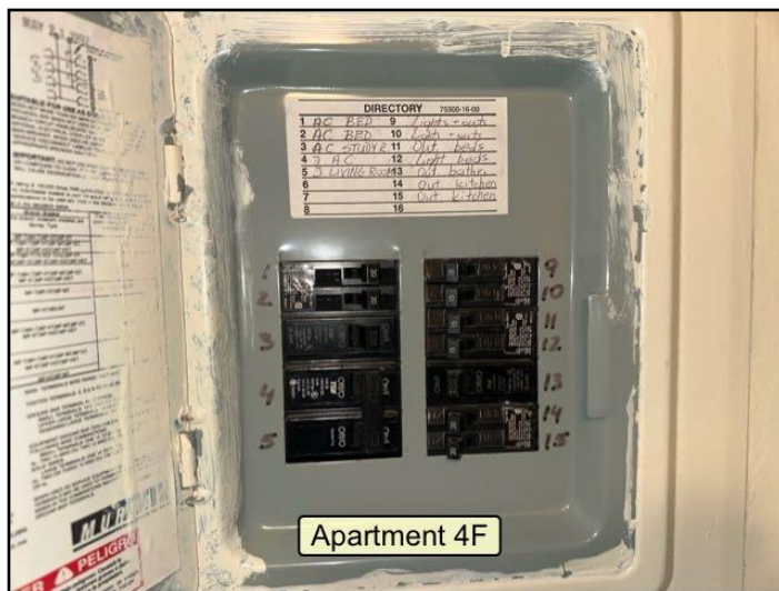
Apartment 4F- Sub panel
