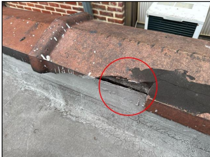
Parapet wall coping damaged
