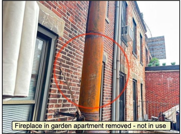
Chimney walls rusting or pitting
