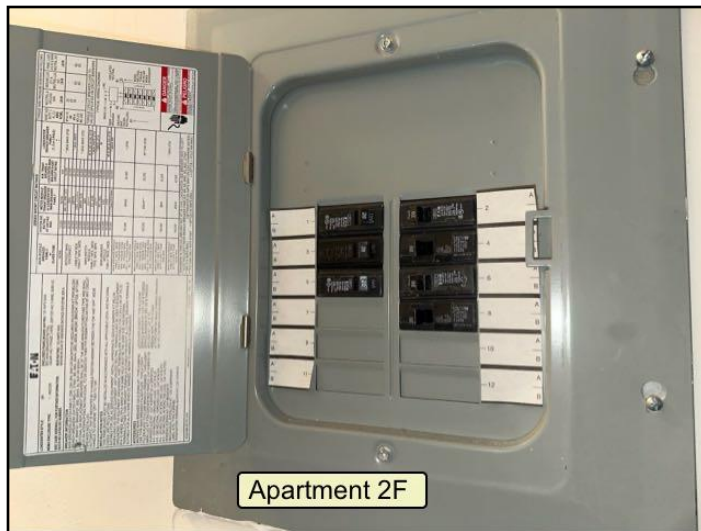
Apartment 2F- Sub panel
