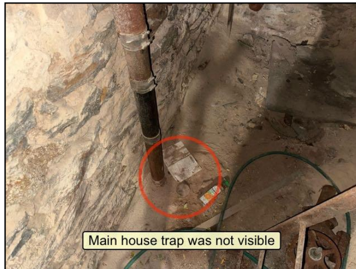
Main house trap not visible
