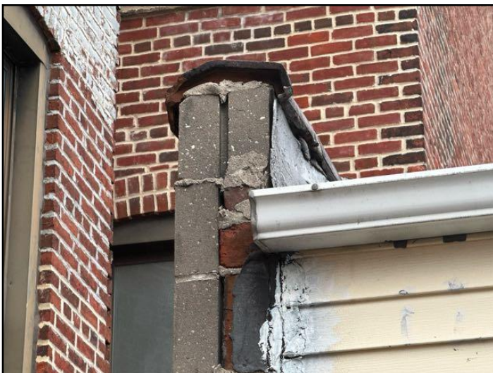
Parapet wall coping damaged
