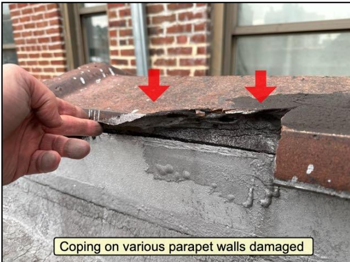
Parapet wall coping damaged
