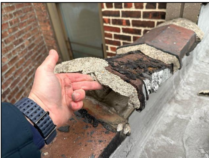
Parapet wall coping damaged
