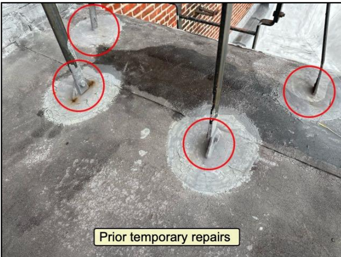
Openings at seams or flashings
