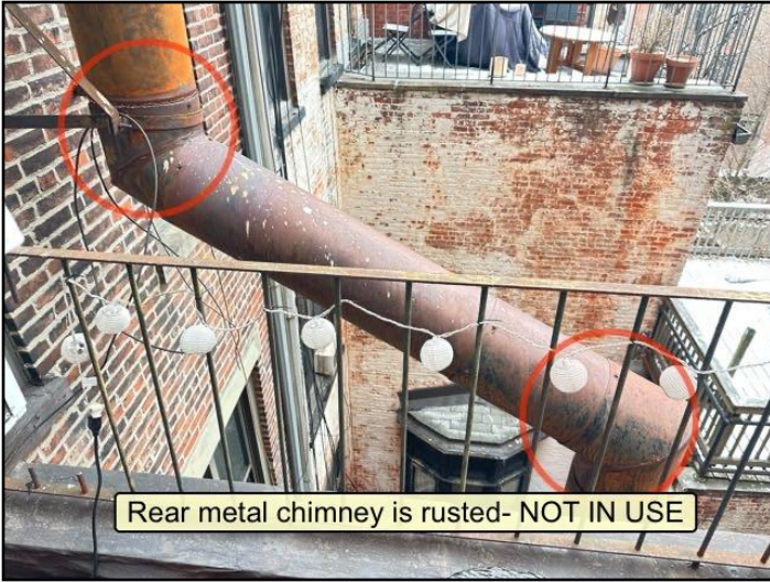
Chimney walls rusting or pitting
