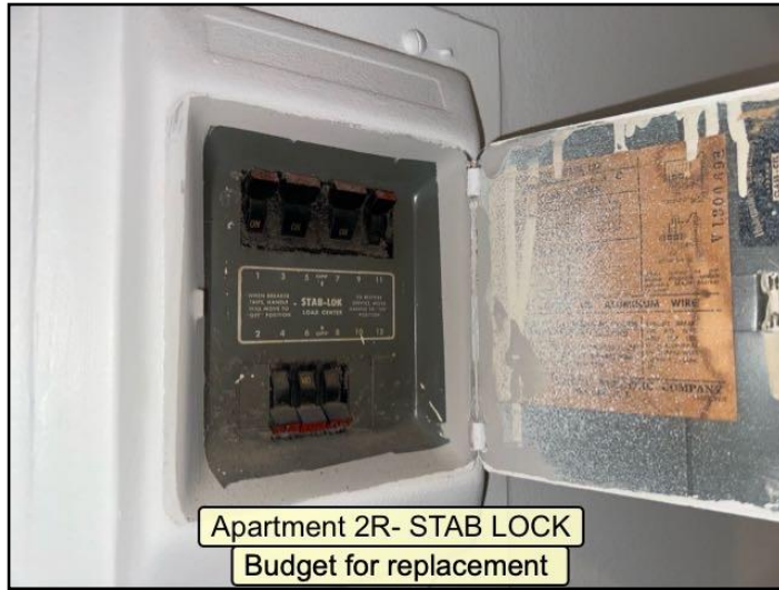
Apartment 2R- Sub panel
