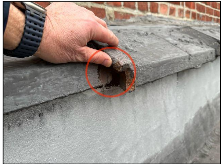
Parapet wall coping damaged
