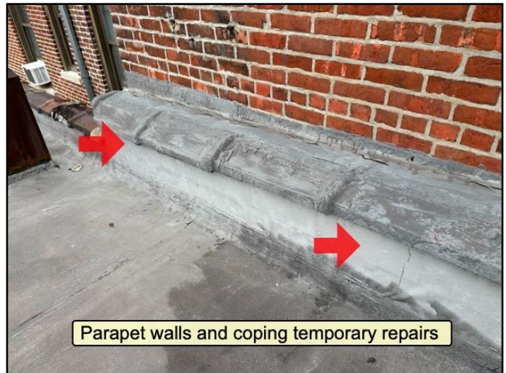
Openings at seams or flashings
