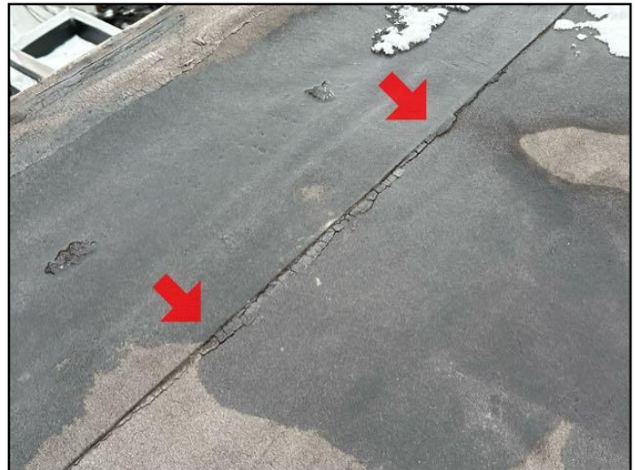
Openings at seams or flashings
