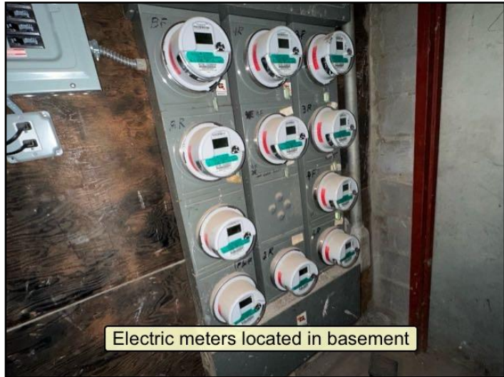
General view of electrical system
