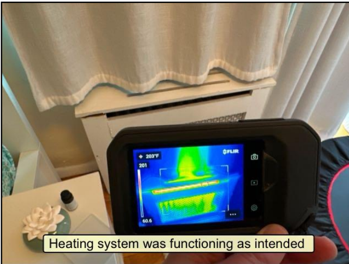
General view of heating system
