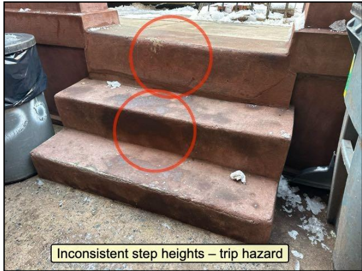
Stair rise too big or not uniform
