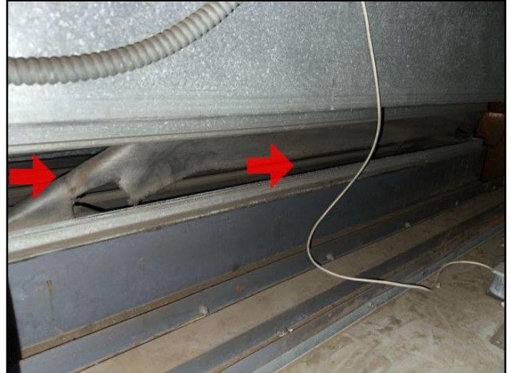
Disconnected or leaking
