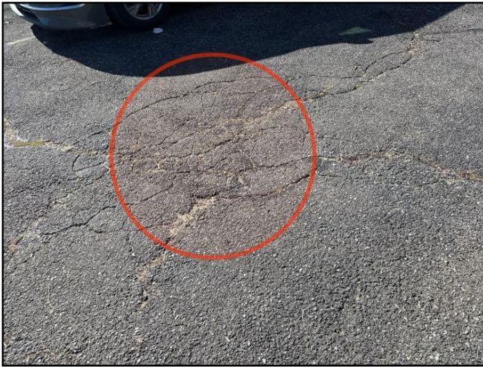
Cracked or damaged surfaces
