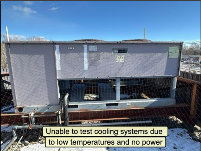
Power turned off
