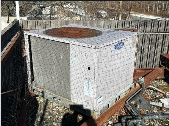
Power turned off
