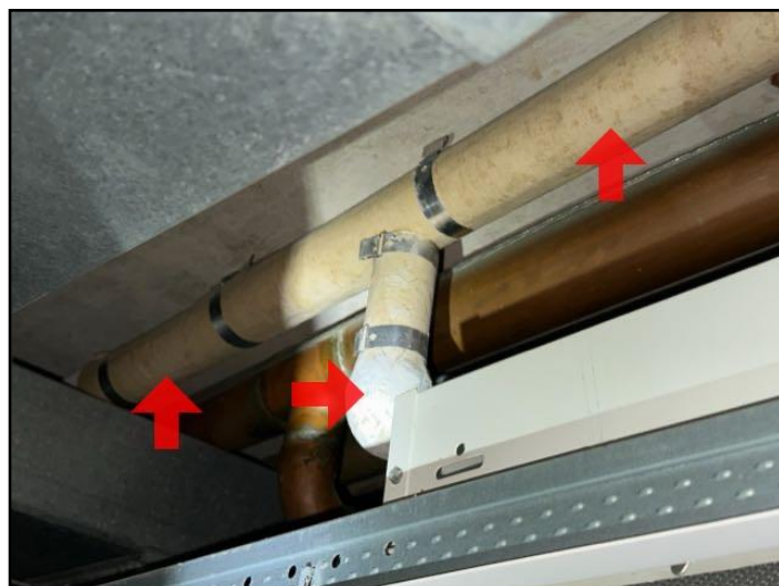
Possible asbestos containing materials
