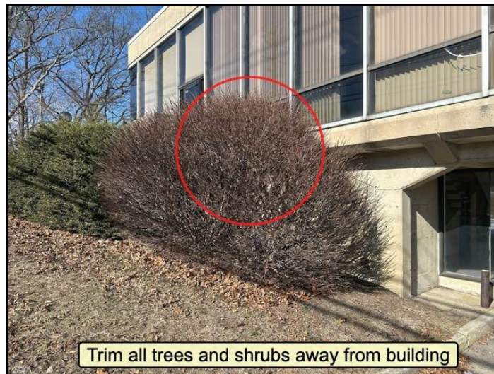
Trees or shrubs too close to building
